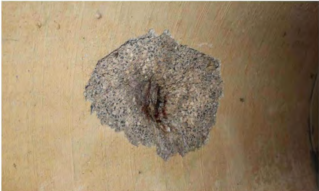
Spall in new section of cell 1
