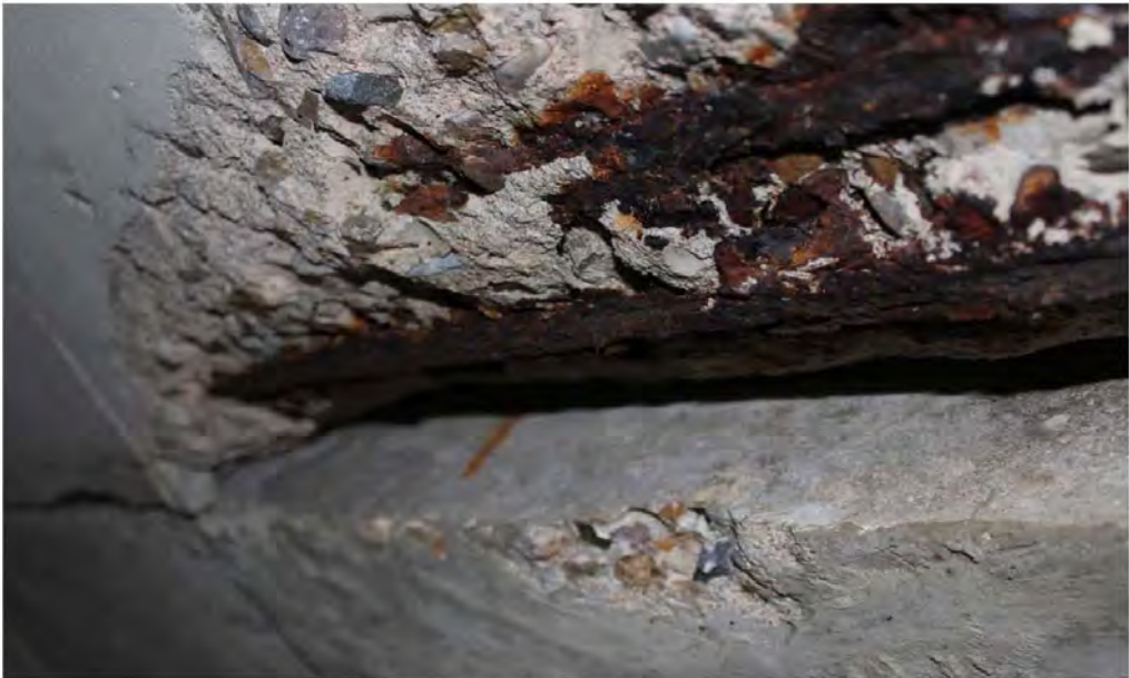
Spall and corroded reinforcement in top of unit 11
