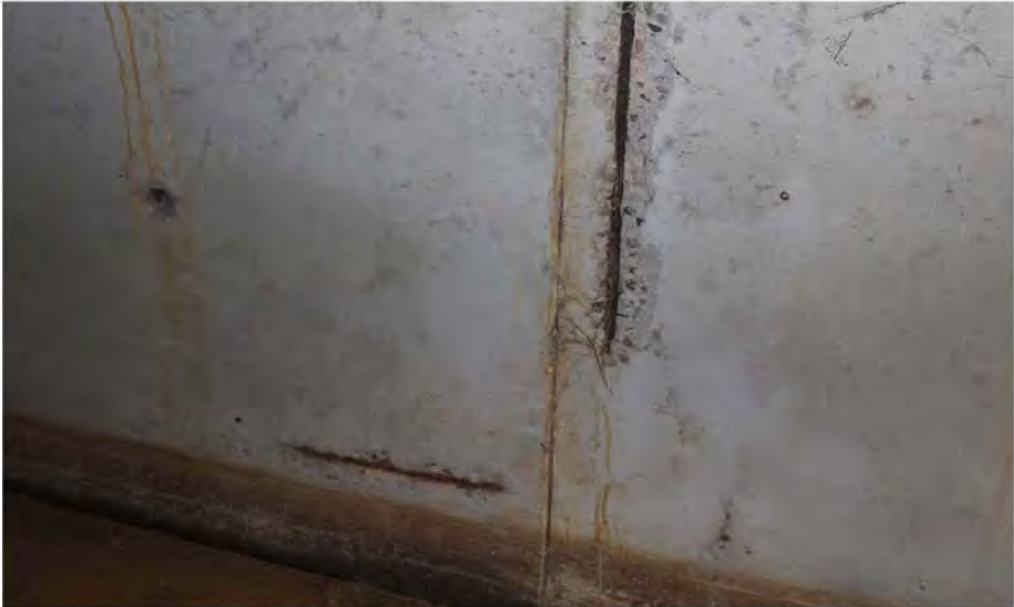
Exposed reinforcement (units 7 and 8 north side)
