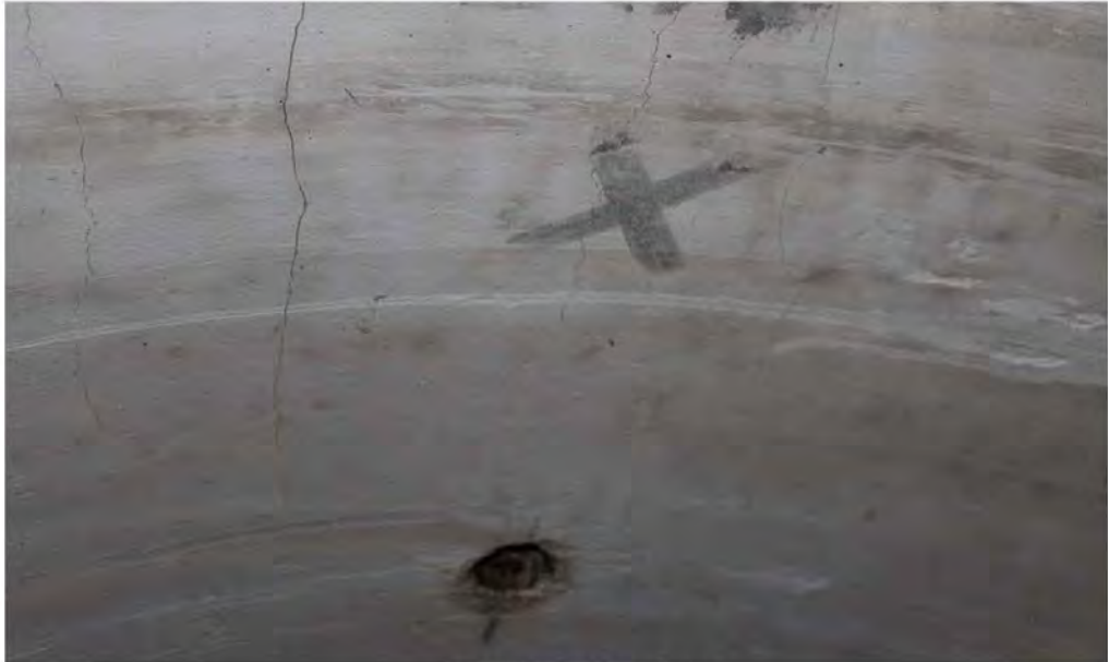
Cracking in top of pipe
