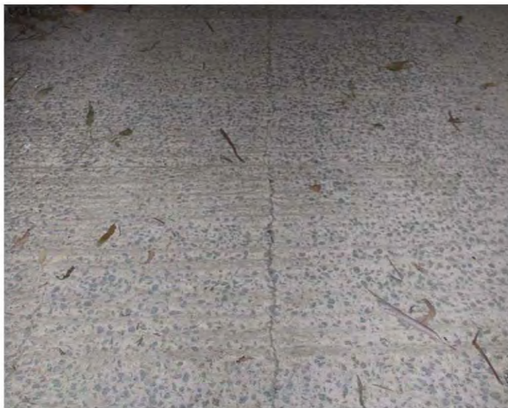
0.3mm crack in base slab
