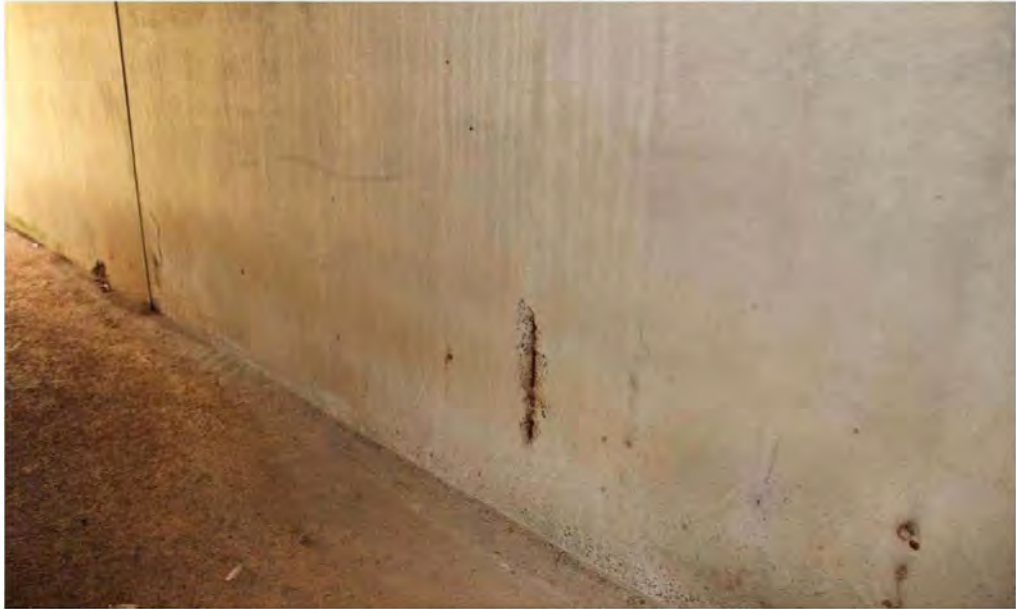
Exposed reinforcement in culvert wall
