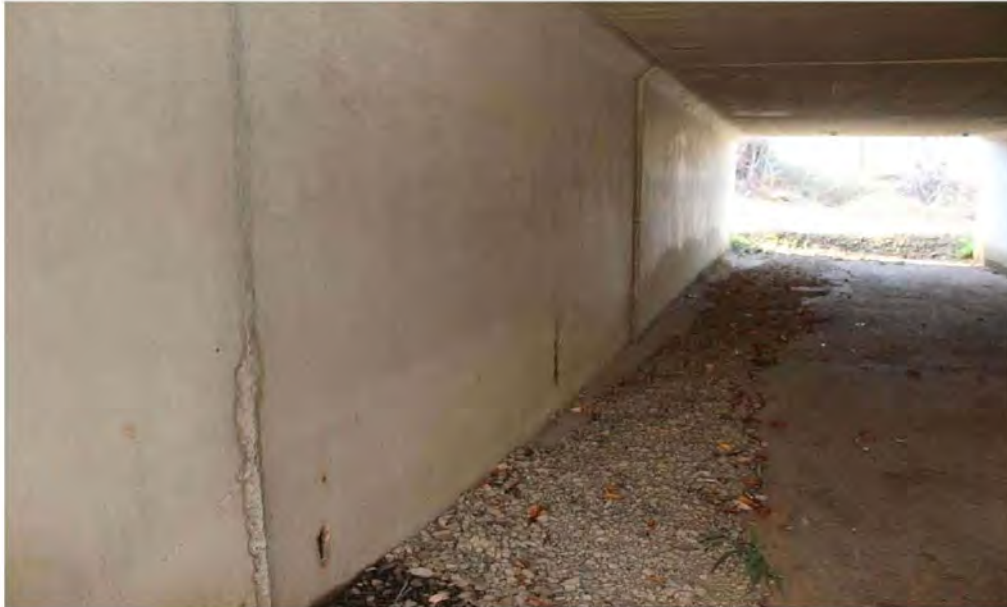
Exposed reinforcement in culvert wall
