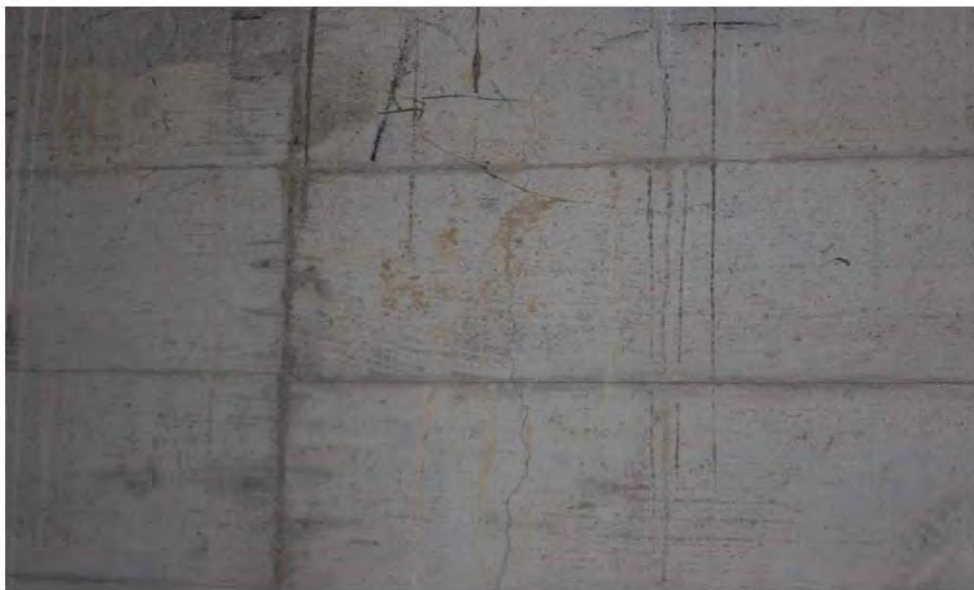
0.1mm vertical crack in Cell 3
