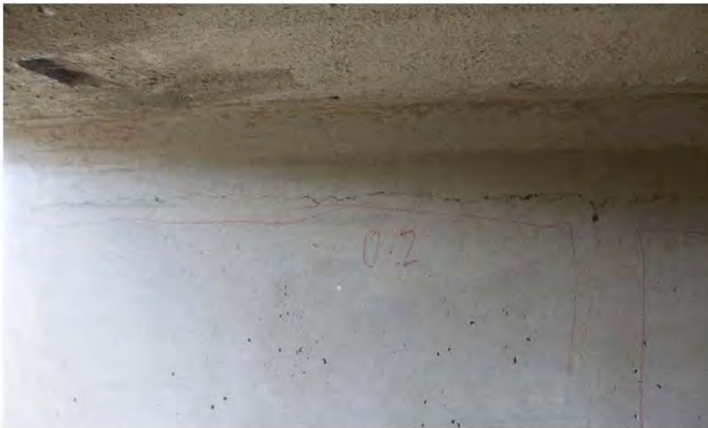
0.2mm horizontal cracking at top of wall and vertical cracking in middle of unit
