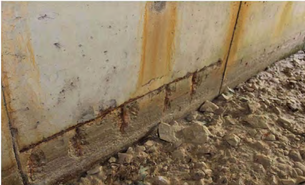
Exposed reinforcement (unit 3 north side)
