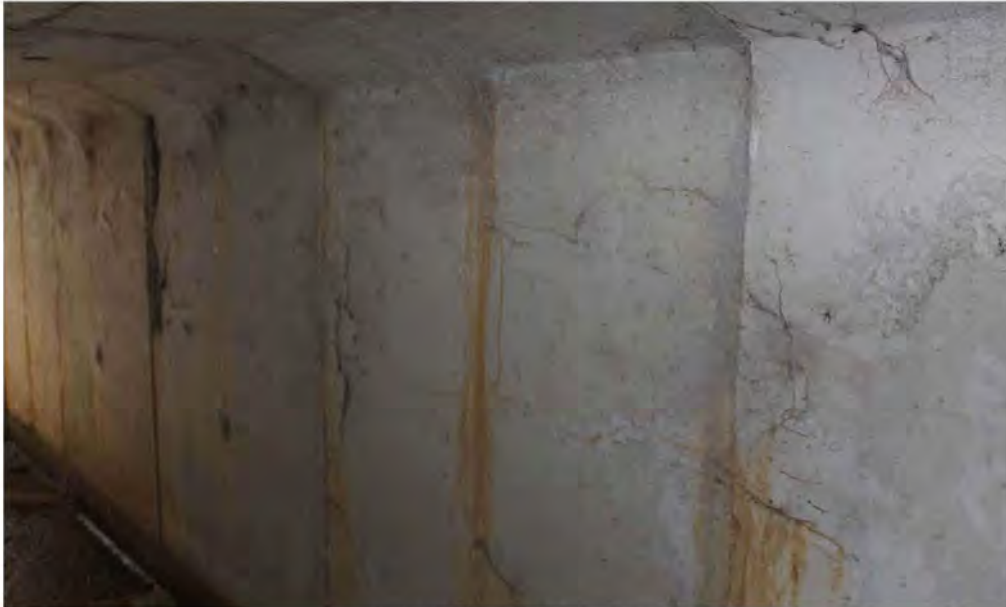
Cracking and spalling on sides of units
