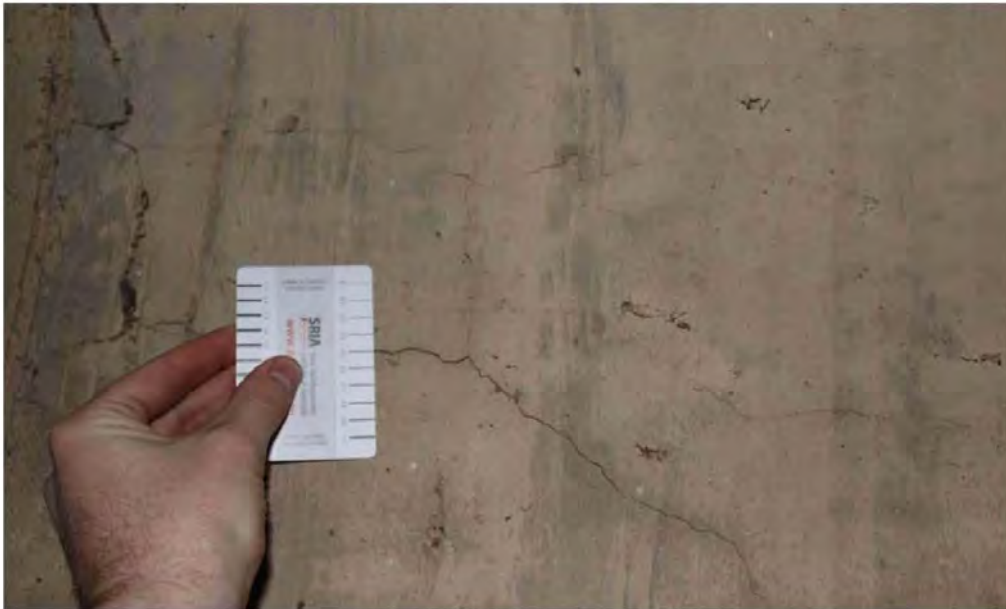
0.5mm cracking in pipe
