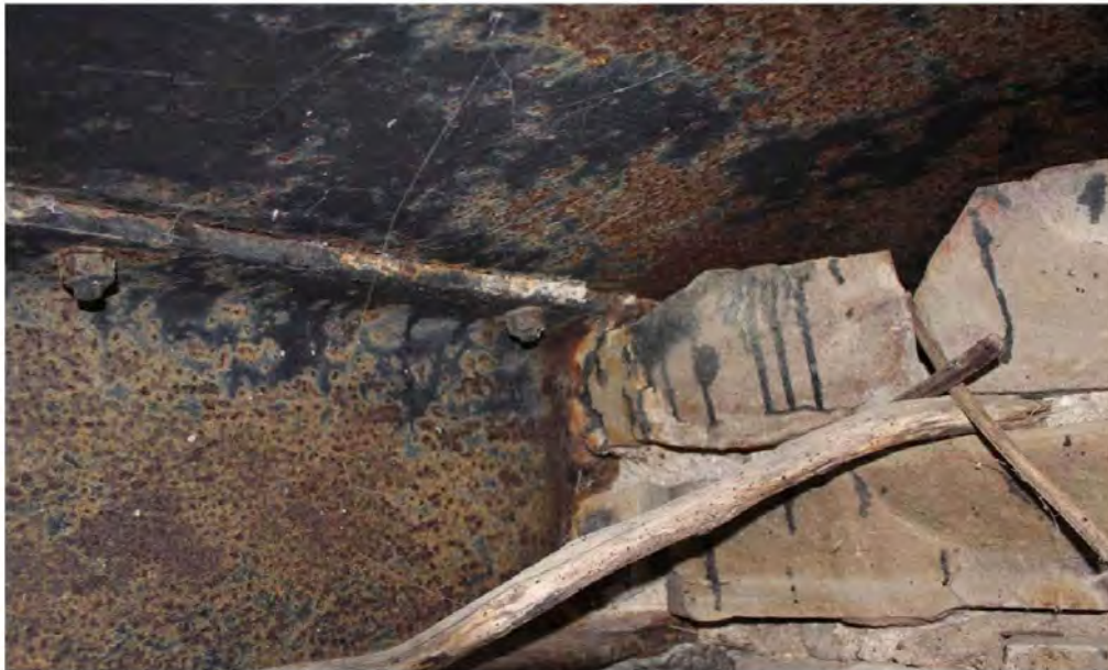
Corrosion of southern end of beam 4
