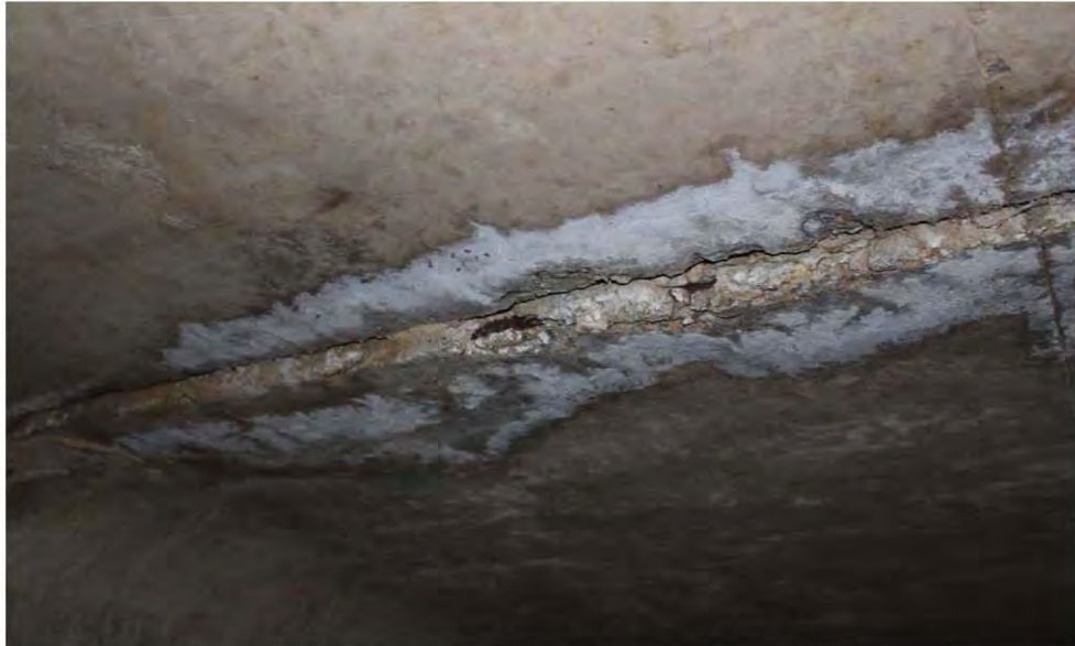
Exposed reinforcement and efflorescence in edge of culvert roof
