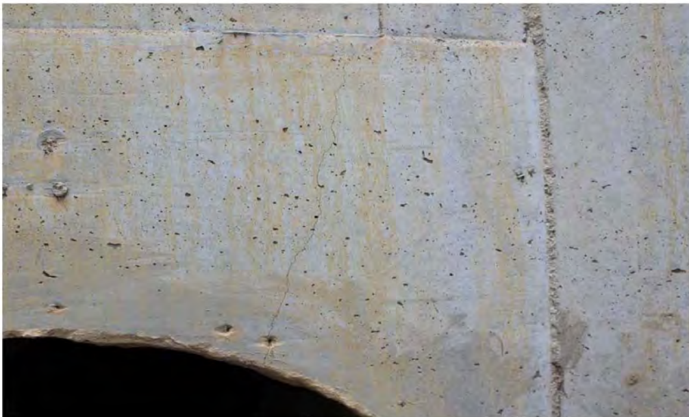
0.3mm crack in headwall at inlet
