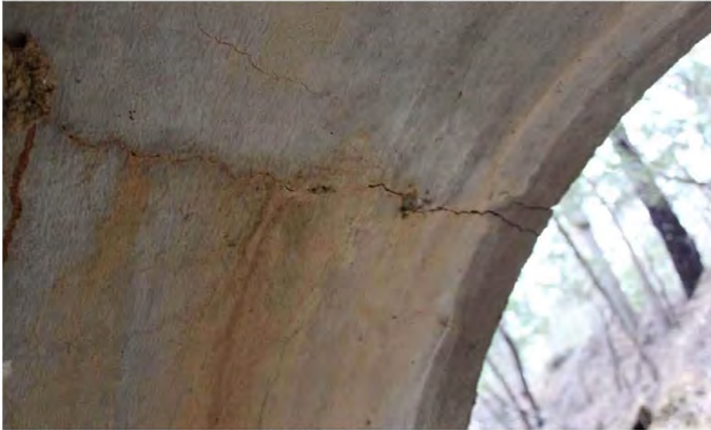
Cracking in side of unit 1 northern side
