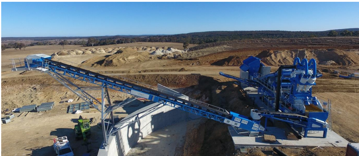
Figure 5 - Assembled sand wash plant
