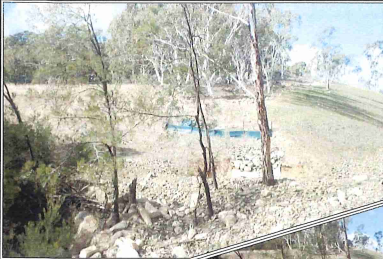
Plate 1: Batter revegetation and sediment fencing adjacent to the Bungonia By-pass, looking east (Ref: E625G_016)
