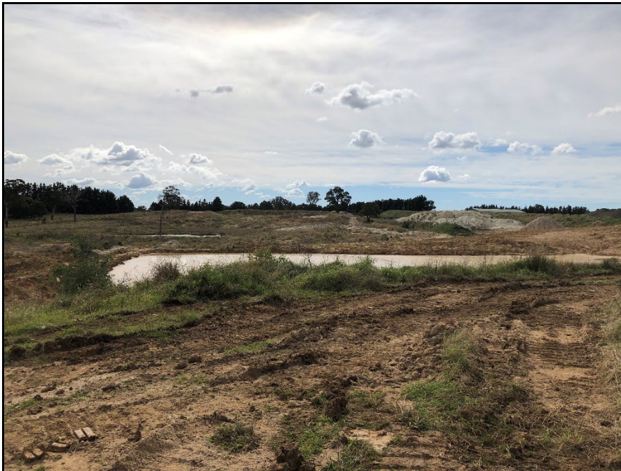
Photo 6: Looking north east across Silt and Oversize Management Area 2. Active Silt Cell 2 in centre of image.
